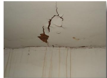
Interior damage to wall and ceiling
