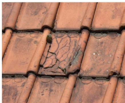
Exterior cracked tiles
